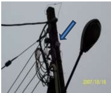
Installation at a Street lamp
